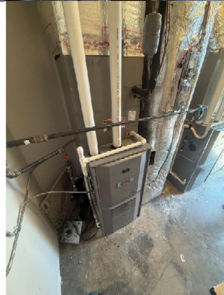
Figure 3: AC-2 Air Handling Unit
