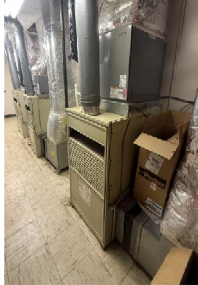
Figure 5: GF-3 Air Handling Unit
